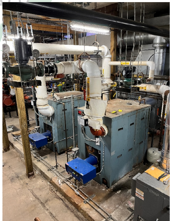
Figure 16: McConnell Center HVAC equipment to be assessed.
