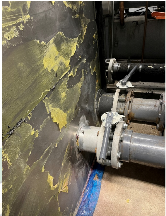
Figure 15: Ice Arena Glycol Tank Leak.
