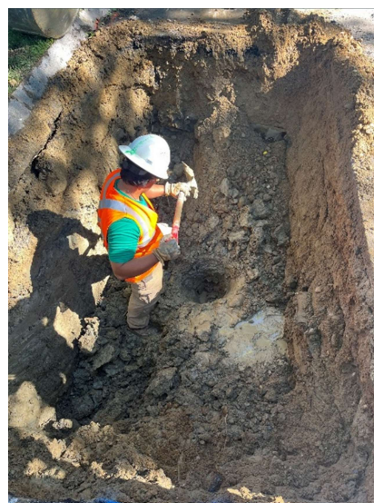
Figure 21: Martin Lane water main break.
