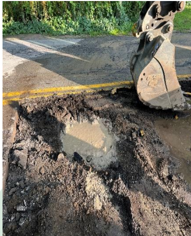
Figure 18: Cochecho - 6" water main
