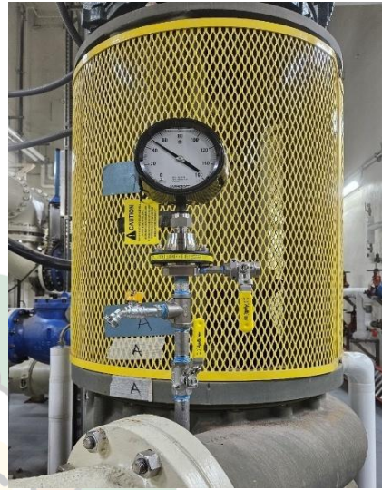
Figure 27: New gauge for monitoring.
