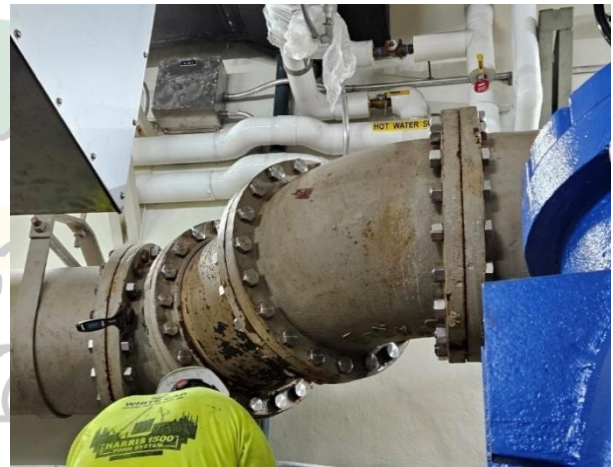
Figure 34: The current nuts and bolts for piping are being replaced with all Stainless Steel.
