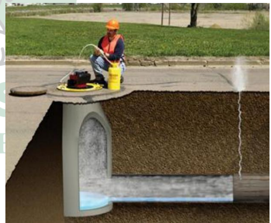
Figure 1: Typical smoke testing setup.
