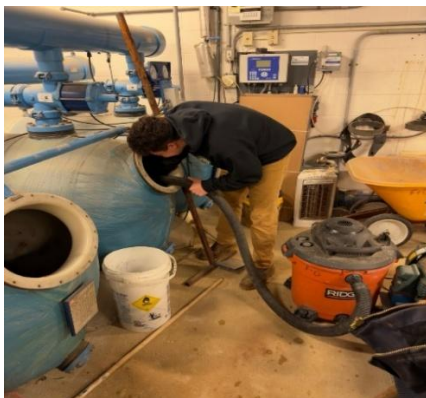
Figure 26: Sand filter cleaning at Jenny Thompson Pool.
