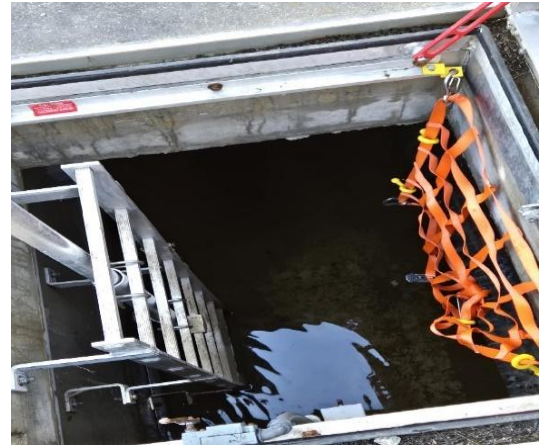
Figure 24: North End Tank Vault
