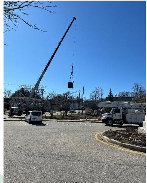
Figure 28: Dover Public Library – Transformer
