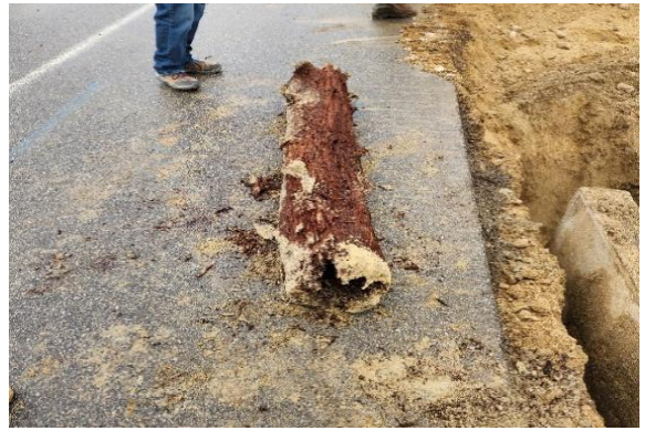
Figure 13: A segment of the old wooden water main from Central Ave.
