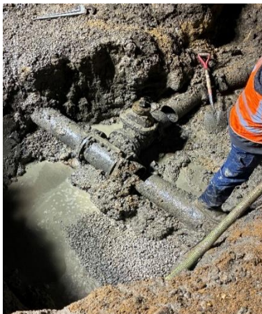
Figure 19: Broken Water Valve.
