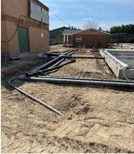
Figure 30: Jenny Thompson Pool – main piping.
