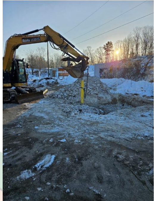
Figure 18: Removal of the old concrete generator pad at the River St PS.
