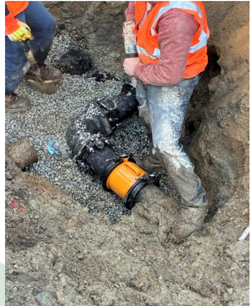
Figure 13: Reconnecting the Main on Back Road after the old tee was removed.
