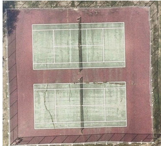
Figure 2: FGH Elementary School Tennis Courts showing signs of severe deterioration.
