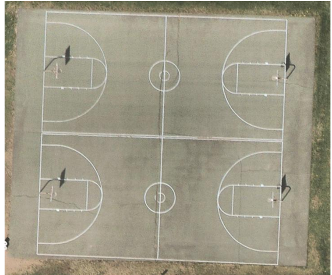
Figure 4: Woodman Park School Basketball Courts with severe cracking and lack of space between courts.
