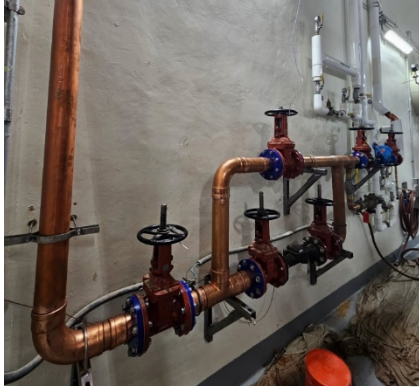
Figure 35: Copper piping throughout.
