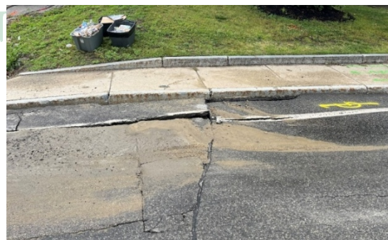
Figure 21: Portland Ave roadway damage before the repairs.
