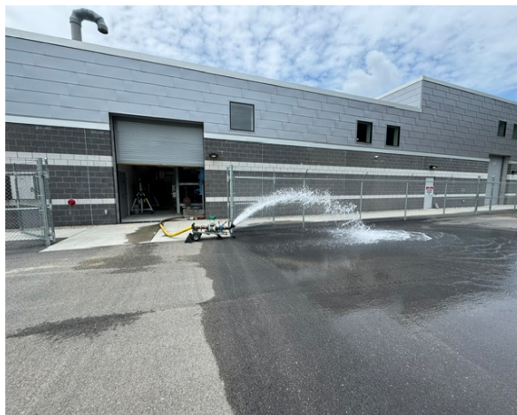
Figure 22: Completed mag-meter calibrations on raw water, finished water, and Bellamy recharge systems.
