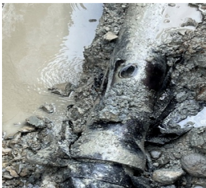
Figure 20: Water main break.
