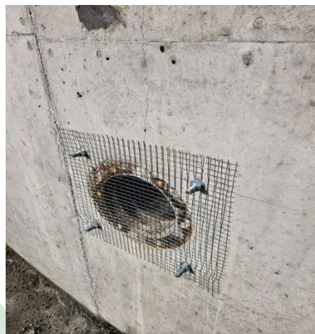
Figure 42: New Screening to prevent clogs.
