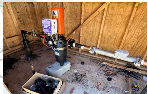
Figure 21: New Pump system.
