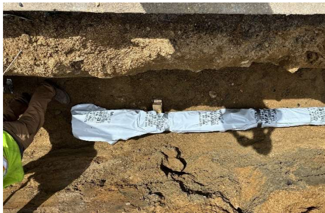
Figure 13: Water main with protective wrap to prevent corrosion.
