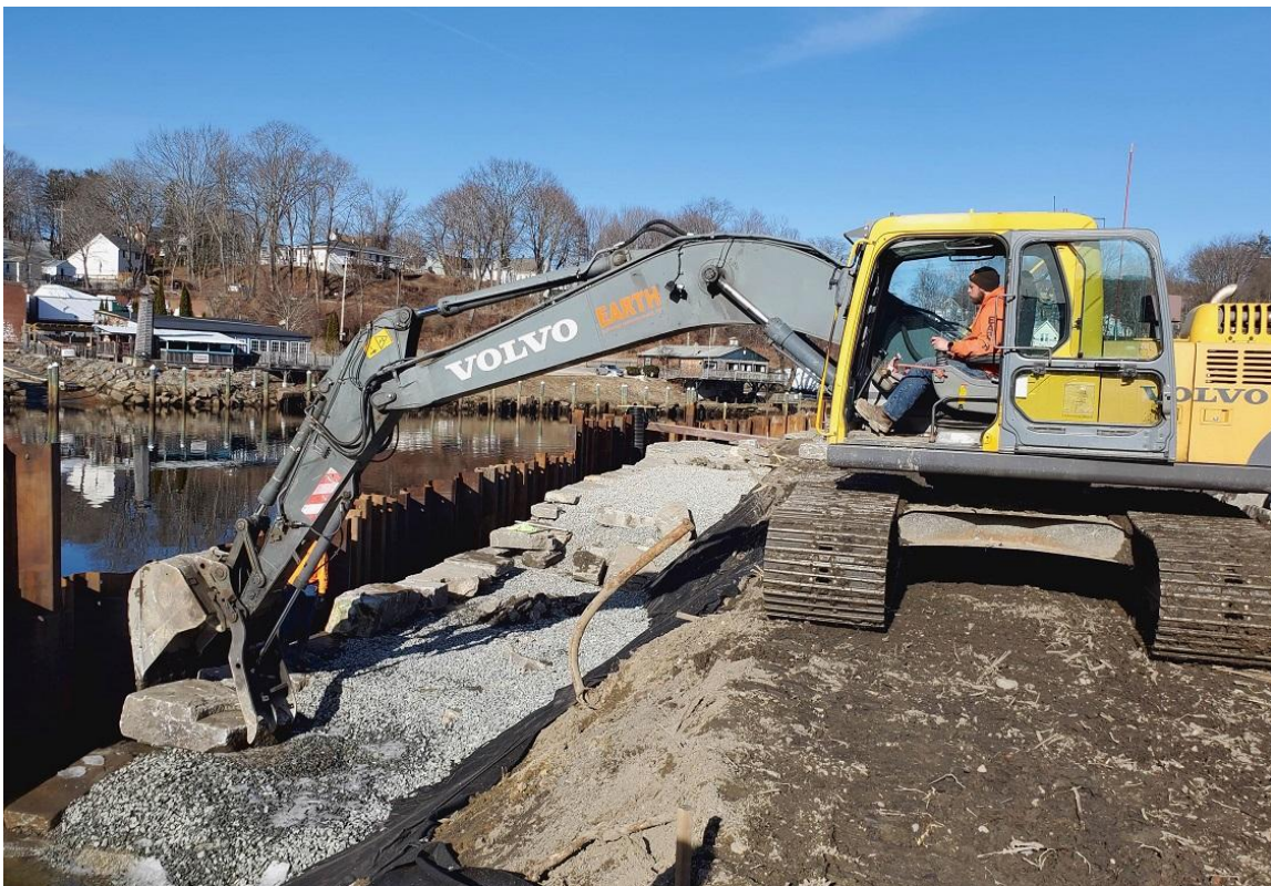
A worker from Northeast Earth Mechanics places a stone on the toe wall.
