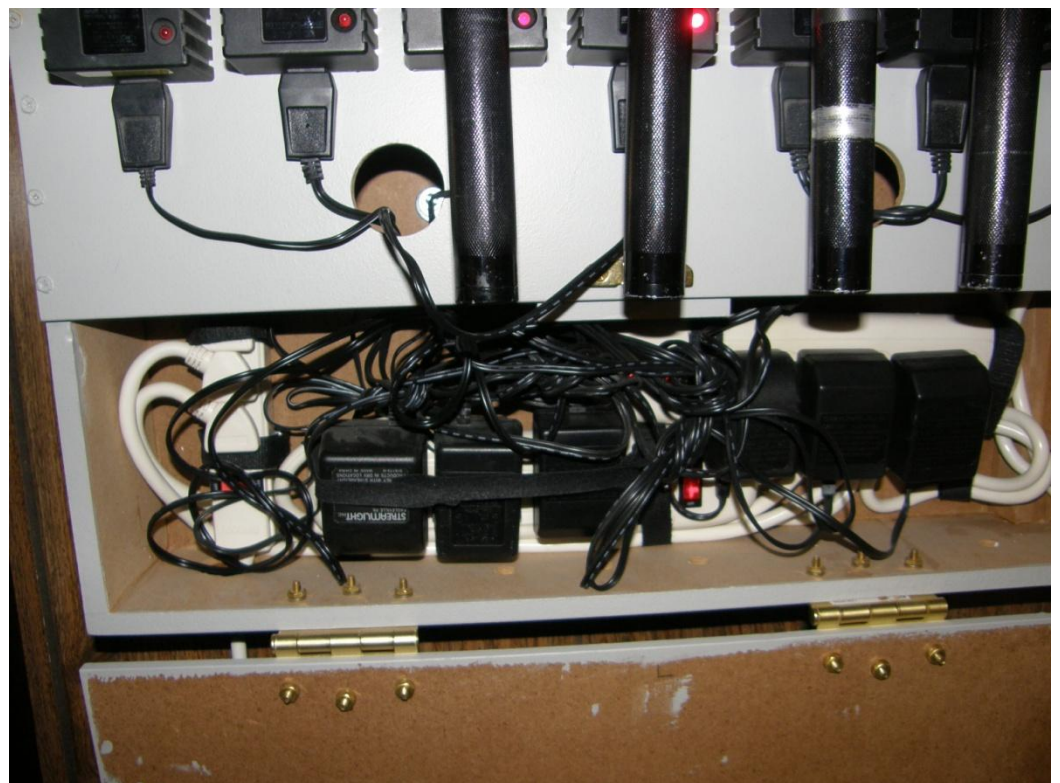
Multiple power strips used to charge flashlights
