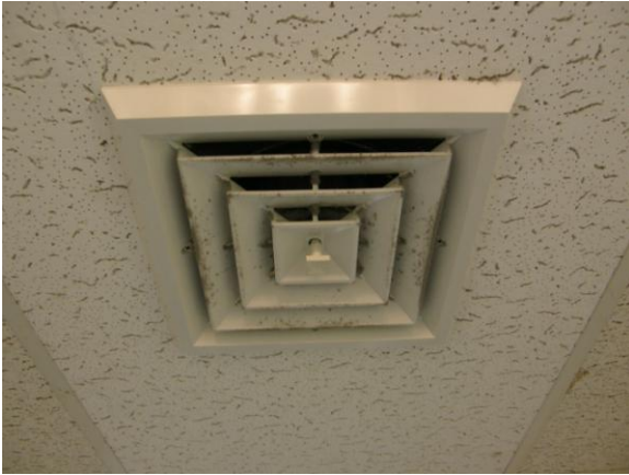
Mold in an air exchange vent in the men's locker room.
