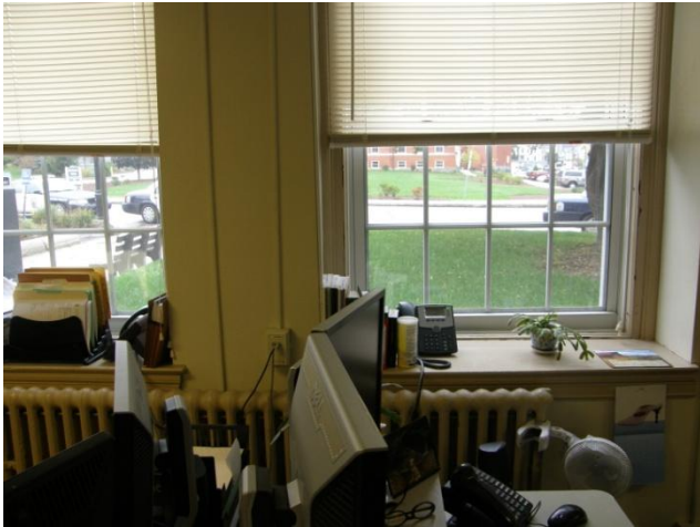
Ground floor windows in the Records Bureau that are not fortified.
