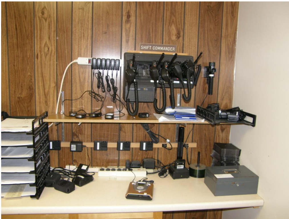
Multiple power strips used to charge portable radios, cell phones and other equipment
