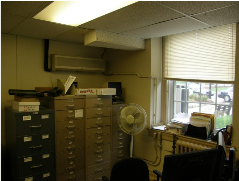
Wall mounted AC unit in Records Bureau office. The AC unit is above records storage that is at risk should the unit leak.
