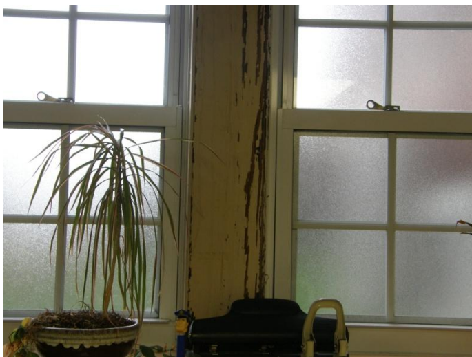
Ground floor windows in the Special Investigations Bureau office that leak and are located above detectives' desks.
