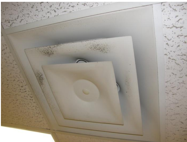
Mold on air exchange vent in Prosecution office.
