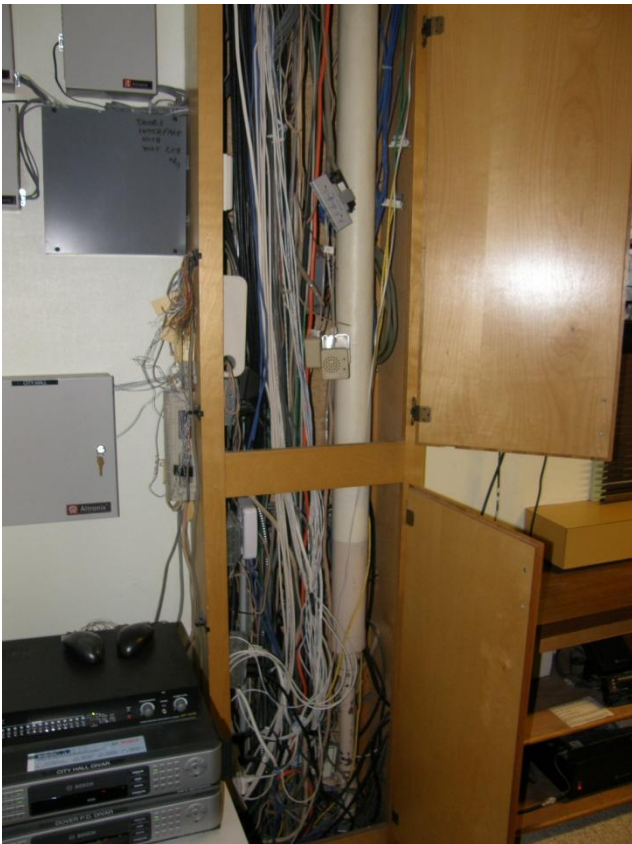
An electrical chase in the Communications Bureau that contains hundreds of wires.
