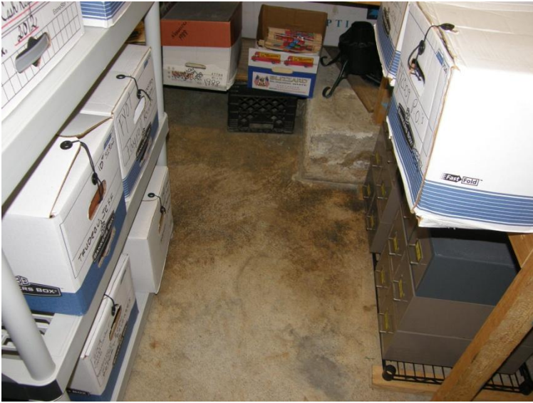
Remnants of gray water flooding in records storage area.
