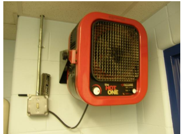
Wall mounted electric heater in the crime lab.
