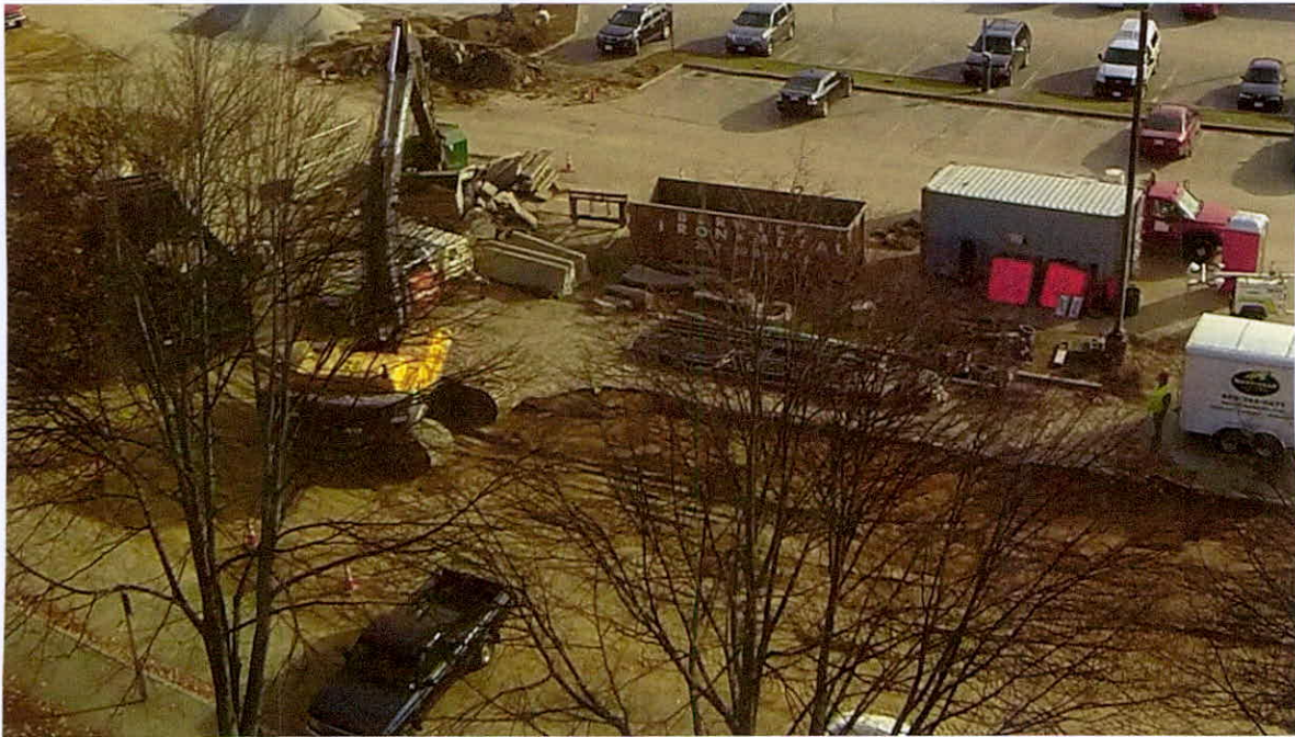
Crews construct the new Orchard Street in the area of the Cochecho Park Building – October 2014.
