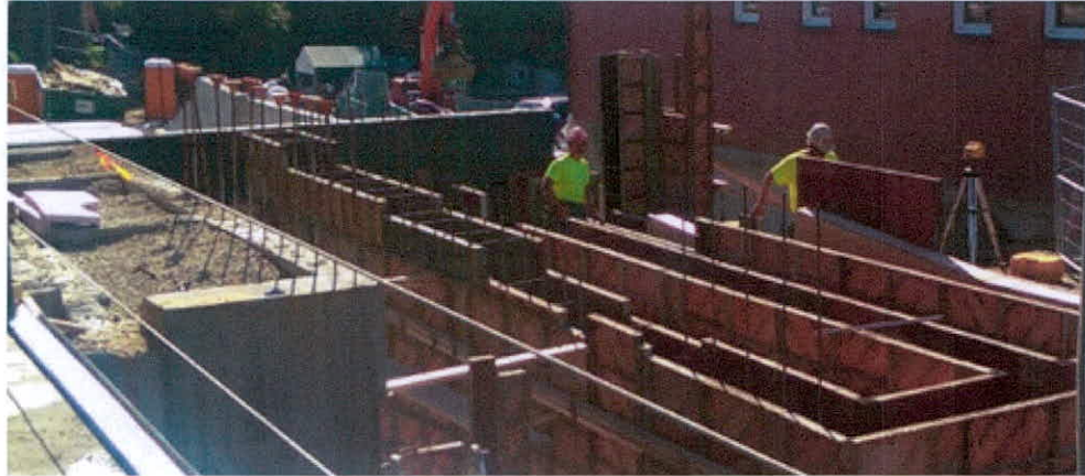
Construction of concrete handicap ramp located in Southwest corner of site- August 2015.
