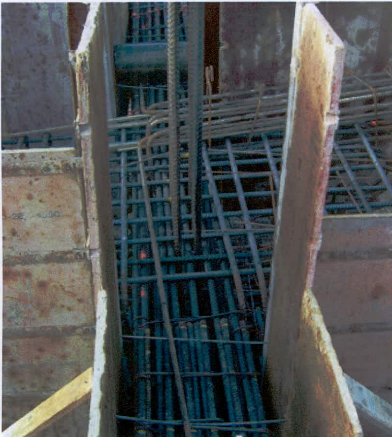
Pile cap and grade beam of footing prior to concrete placement – April 2015.
