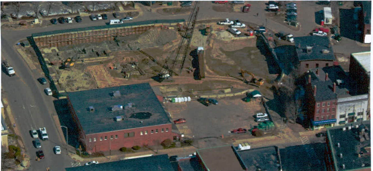
Aerial view of site showing north excavation and new layout of Orchard Street – March 2015.
