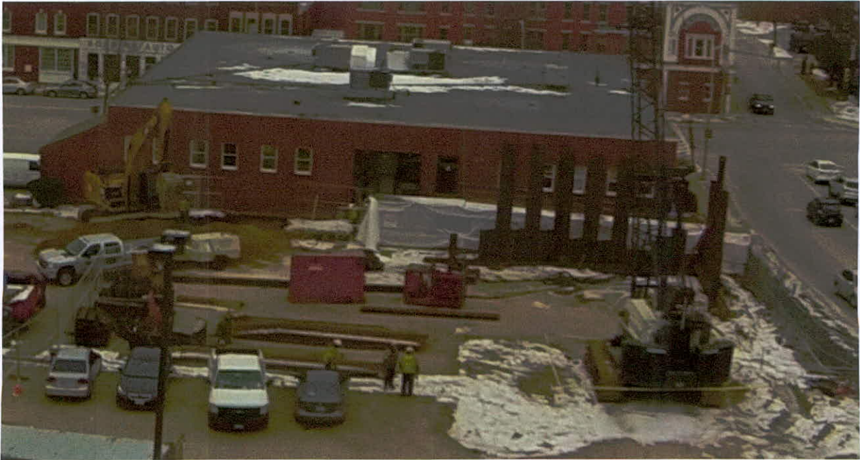
Vertical excavation support piles are installed on the South side of the building lot – December 2014.
