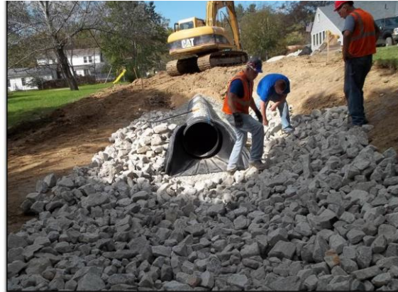
Stormwater management techniques in Dover [Source: Dover Public Works]
