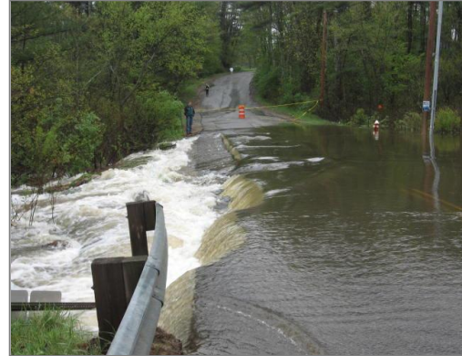
Flooding 2007 [Source: City of Dover]
