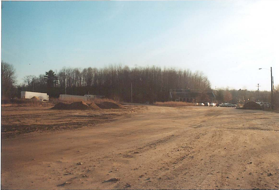
An overview of the subject site looking southeast. The photographer is near the center of the property, the Cocheco River is to the right.
